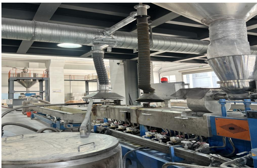
废气收集管道和集气罩
